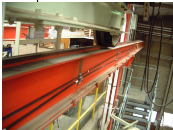
Crane Girder Deflection
